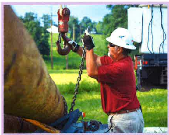
Wayne Prewitt of the Winchester Service Center works to lift a transmission pole.
