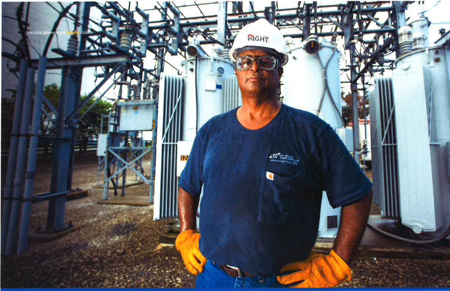
Substation Technician Xenia White and his co-workers in Power Delivery and System Operations nearly matched EKPC's all-time record for system reliability in 2016.
