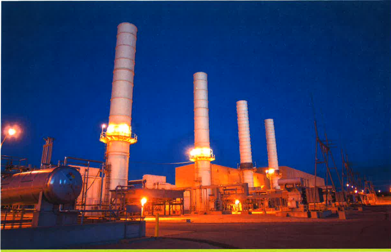
Located on the Kentucky River at Trapp, J.K. Smith Station has nine combustion turbine units. The plant is named after one of EKPC's founders, who spread the benefits of rural electrification across the nation and to countries around the world.
