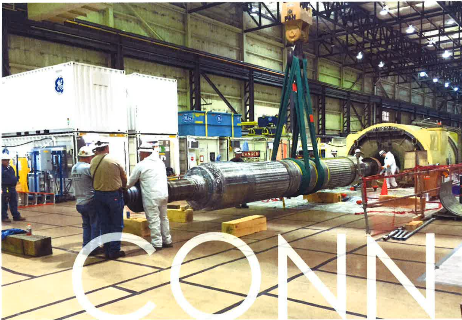
Employees remove the generator field rotor of Spurlock Unit #2 as part of the largest maintenance outage in the history of the cooperative.
