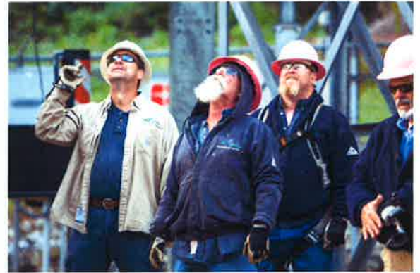
Top: Power Delivery employees set a transformer at the Prestonsburg Substation in October. Employees wore pink hard hats that month in honor of National Breast Cancer Awareness Month. Left: Beth Willoughby serves as a system operator in EKPC's Market Operations Center in Winchester, Ky.
