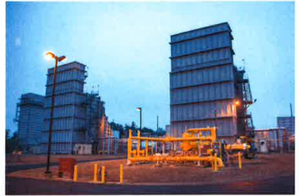
Top: By adding Bluegrass Generating Station, EKPC increased overall capacity 20 percent. Left: Ben Eickbush, left, and Richie Gulley are both plant operators at Spurlock Station.
