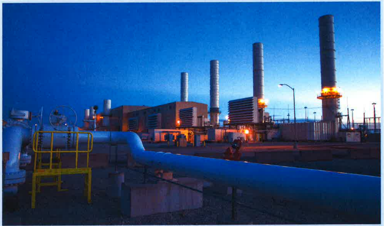
Smith Station in Clark County has nine natural gas fueled units that help EKPC to meet peak system demand.
