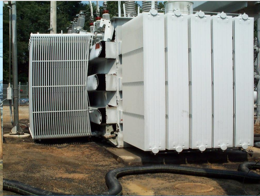
230 kV Transformer Failure in 2001
